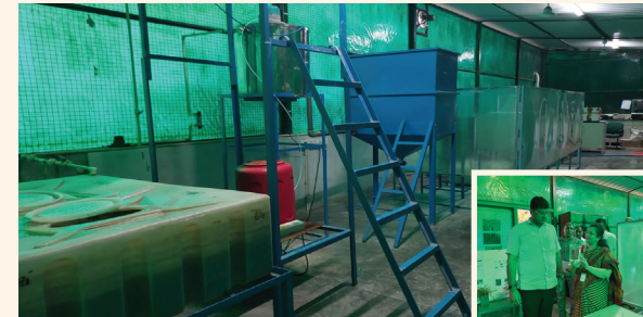
10 KLD tadox ® WWT plant treating mixed sewage in TERI, Gurugram since Aug. 2020; Visit by Dy CM Haryana
