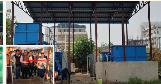
20 KLD tadox ® WWT plant in Textile CETP, Kanpur under 'Namami Gange' Program; Inauguration by DG NMCG.
